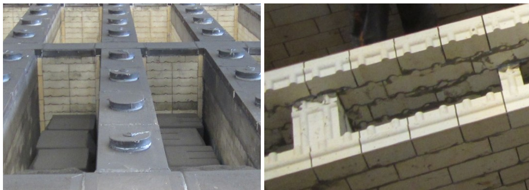
Figure 1: Anode baking furnace. Left: pits loaded with anodes, Right: top of flue wall under construction.
